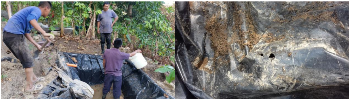
Figure 3 – Old cisterns. Left: construction in 2014. Right: damaged cistern in 2017
