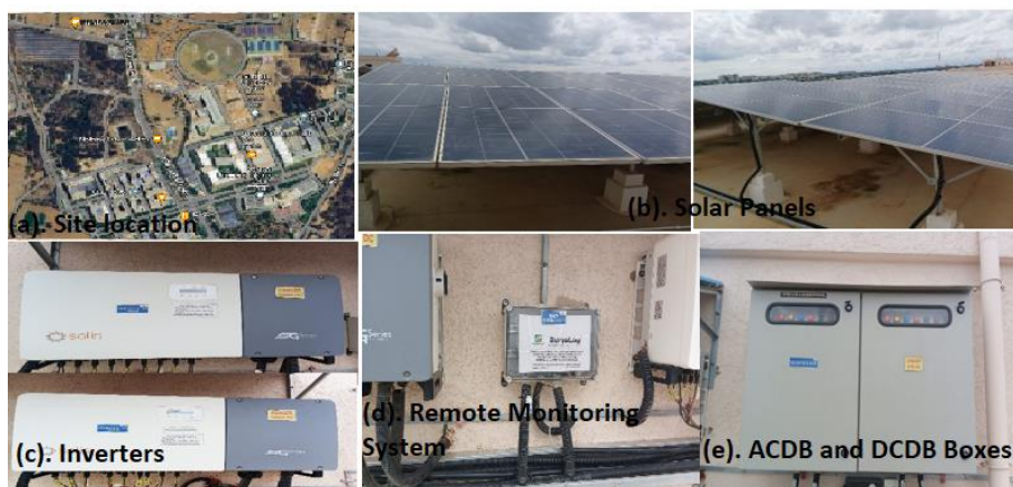
Figure 3. MUJ installed 800 kWp solar power plant photo
